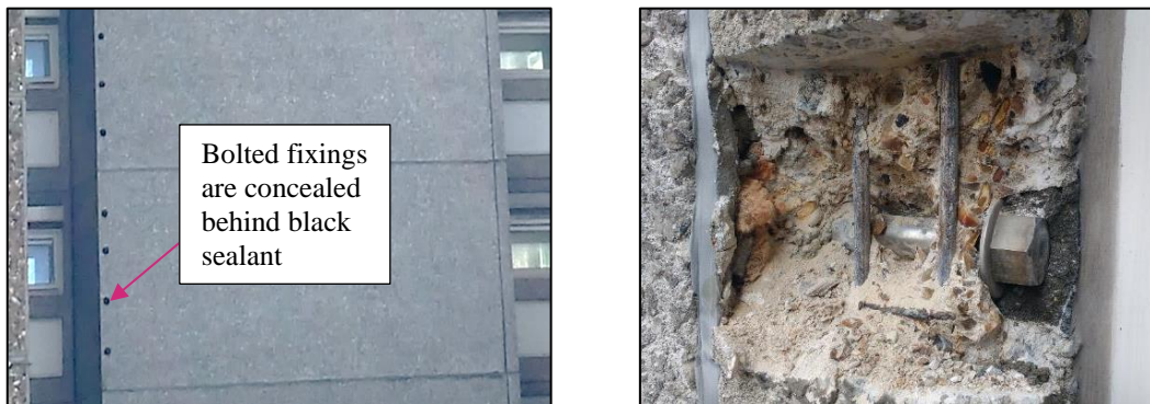
Figure 10 Fixings bolts are concealed behind black sealant (LHS). Fixing bolt exposed by breaking away surrounding concrete (RHS)
