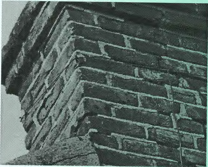
Figure 2.2 Leaning chimney stack and perished mortar pointing typical of sulphur attack.
