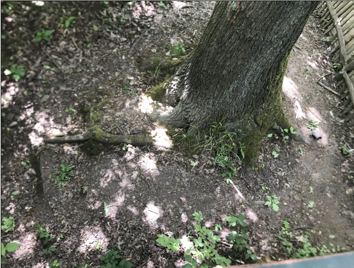
Photograph 2: Root architecture trending away from abutment with surface root running parallel to it
