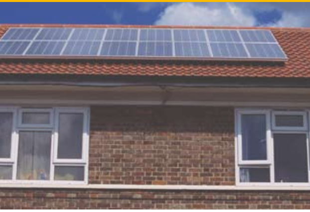
A roof mounted solar panel © third-avenue.co.uk
