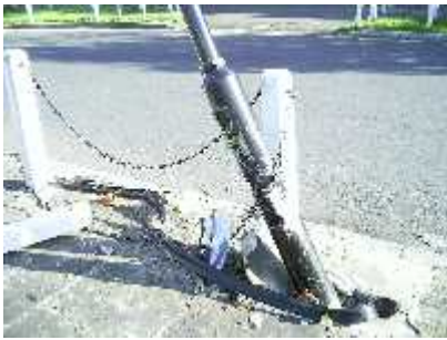
It looks bad and might be dangerous
